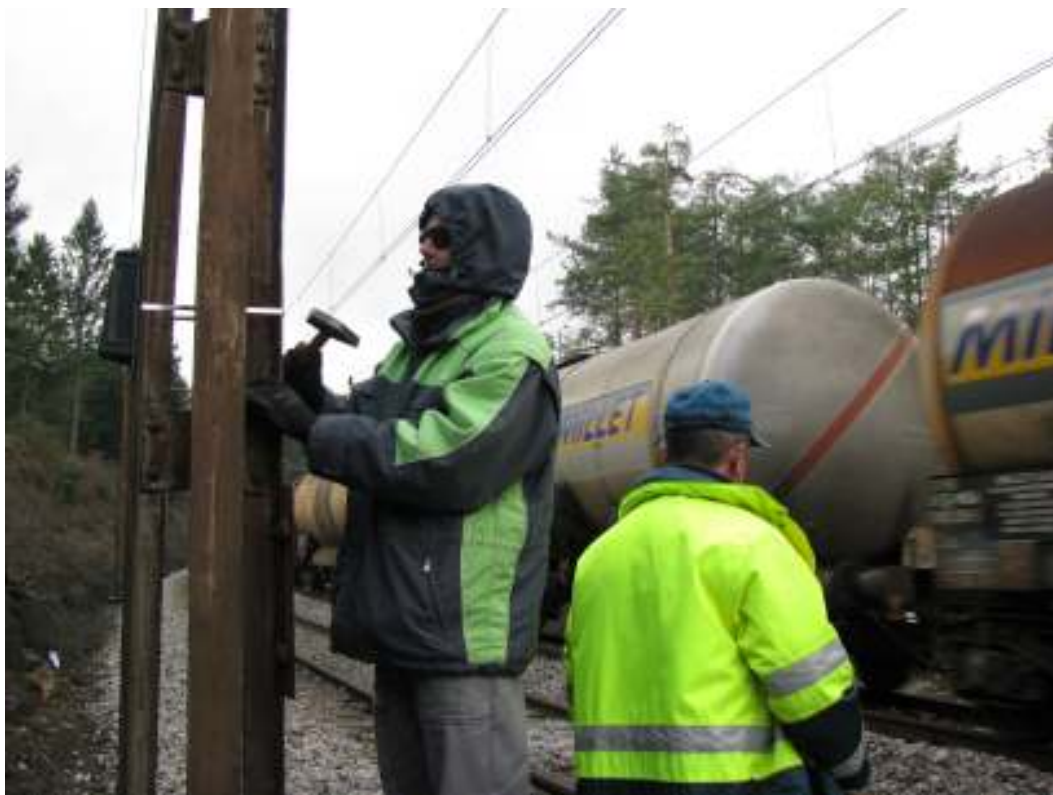
Figure 4: Installation of acoustic deterrents on electric poles along railway sections (photo: M. Zaluberšek, 2015).
