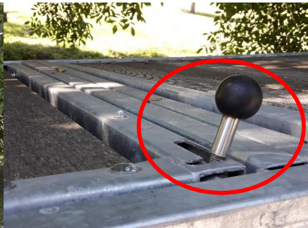
Figure 8: Cover pin was only partially closed.
