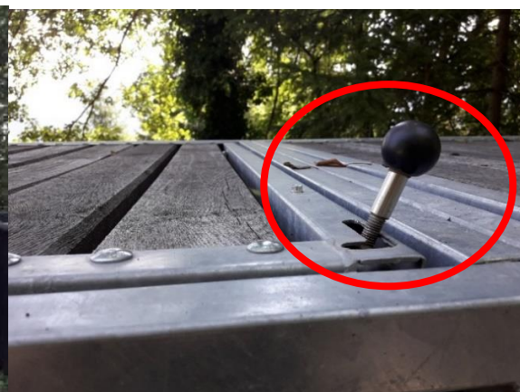
Figure 15: cover pin in not properly locked.
