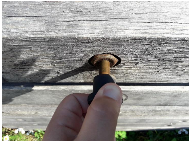
Figure 11: Slightly rusted, but operating cover lid.
